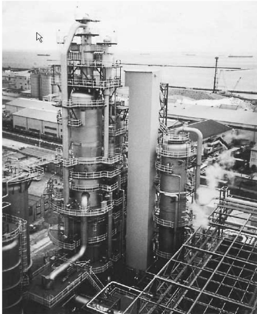
FIGURE 3.4.1 SWI-IFP RFCC unit located in Japan. Photograph shows second- and first-stage regenerators and main fractionator. Note the external cyclones on the second-stage regenerator.
